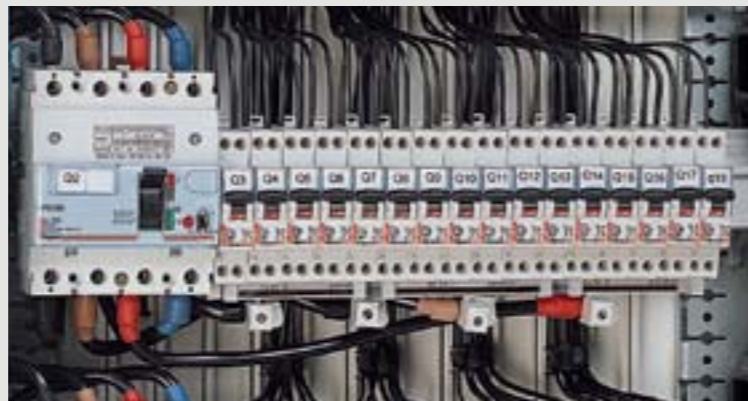
Row of single phase outputs supplied via a DPX 125 (100 A)
